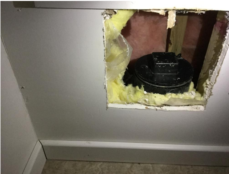
Figure 7: The stack may be hidden behind drywall or under fillings. It is the customer's responsibility to locate and expose it. Relieving a choke from a stack is difficult; Water Services crew will determine the feasibility of doing so.
