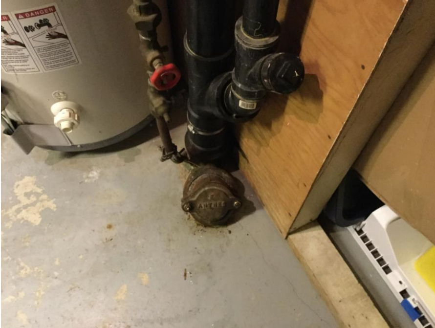
Figure 6: Here is another example of a stack. The stack usually protrudes prominently above ground level.
