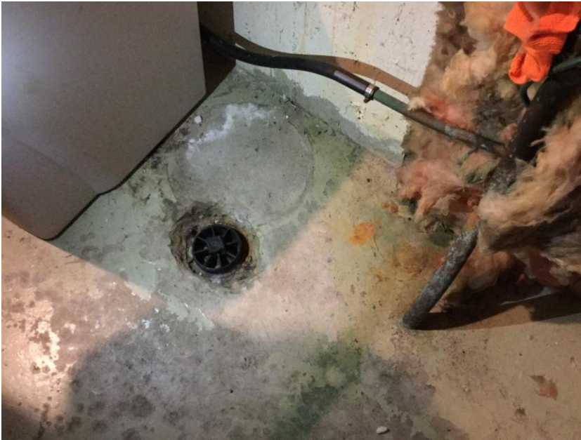
Figure 4: The cleanout may be in close proximity of the entrance of the water line as shown here
