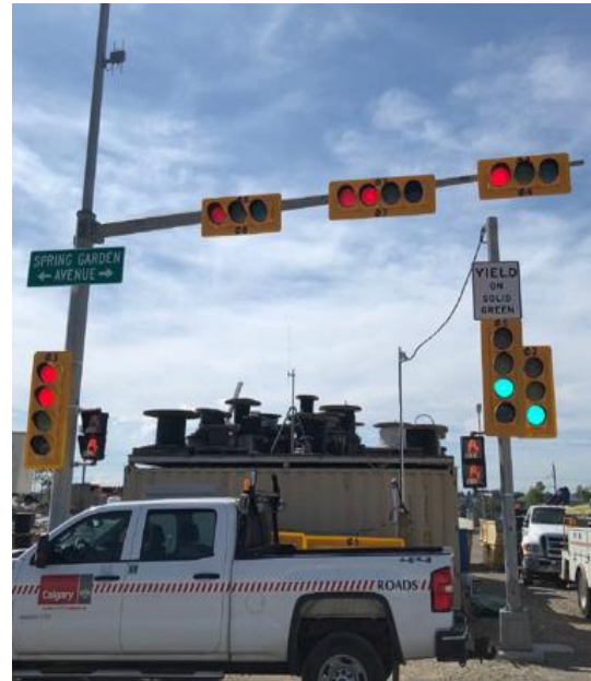
Figure 21: Roadside Equipment Installation at Test Lab
