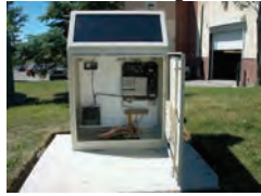
Solar Powered Irrigation
