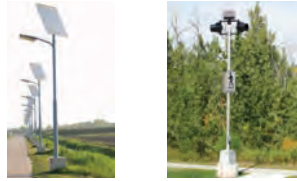
Energy Efficient Lighting
