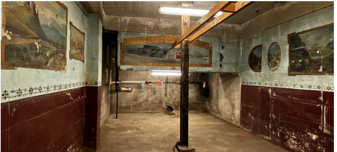
Historic paintings in fire hall basement to be conserved.
