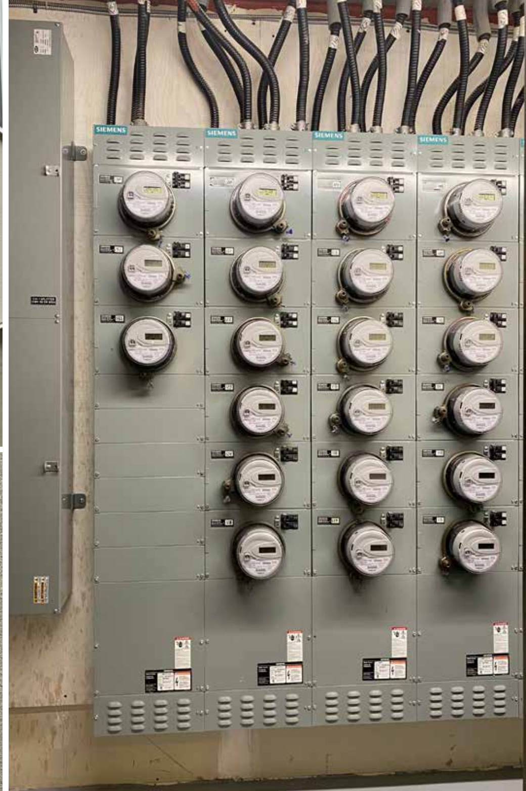
Meter stacks in an electrical room of a multi-residential building.
