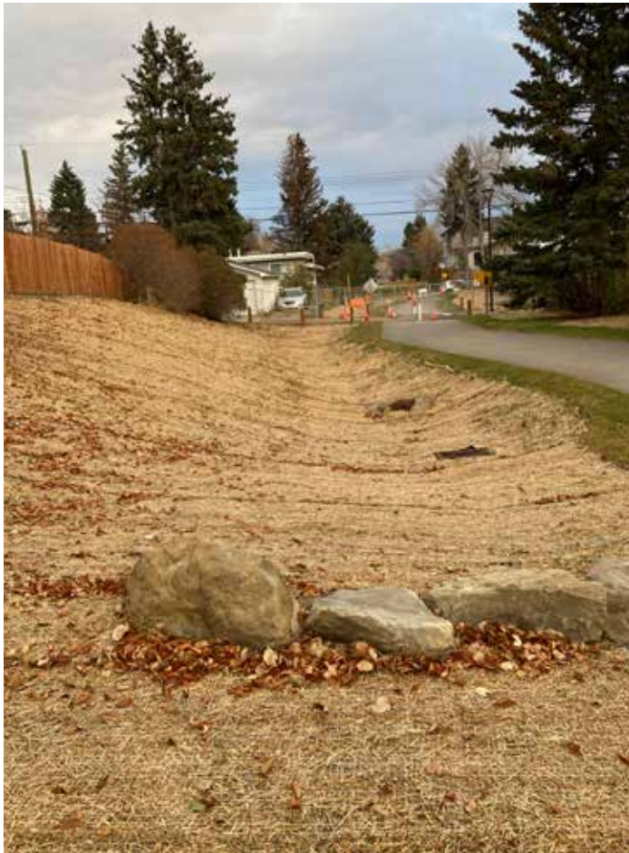
Capitol Hill curb inlet and naturalized swale.
