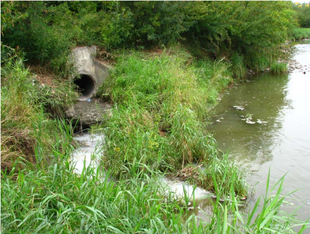
Figure 5. Untreated urban runoff entering Nose Creek (Credit: AMEC / Cows and Fish)
