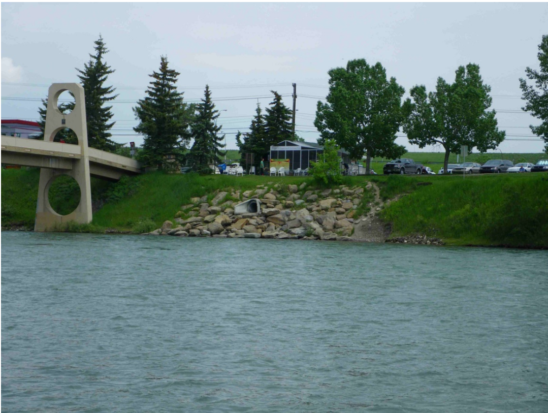
Figure 6. Example of extensive erosion protection works protecting outfall structures on the Bow River (Credit: AMEC / Cows and Fish)
